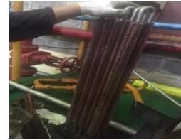
Gambar 2.2 Heat Exchanger (sumber dokumen frengki,2019)
