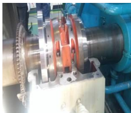
Gambar 2.1 Turbine guide bearing (Sumber Dok frengki, 2019)
